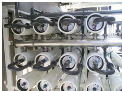
Reverse-osmosis Equipment in a Desalination Facility
