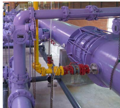
Water Recycling Facility
